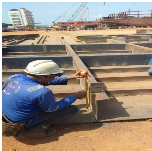
Gambar 2. 43. Timbang Main Deck
