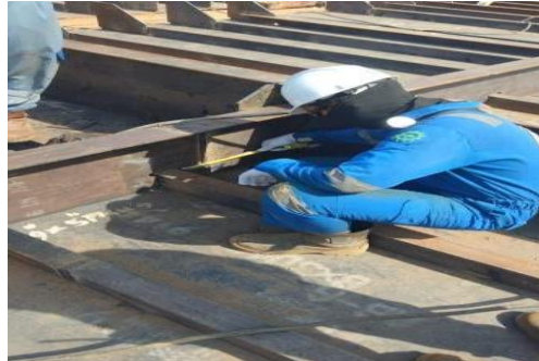
Gambar 2. 42. Fit Up T.Bulkhead
