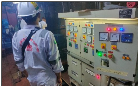
Gambar 2.67 : electrical control engine room
