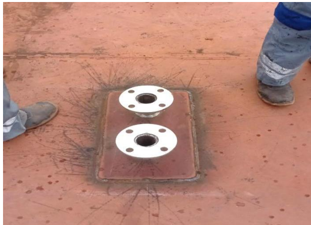
Gambar 2.18 Inspection pipe heating
