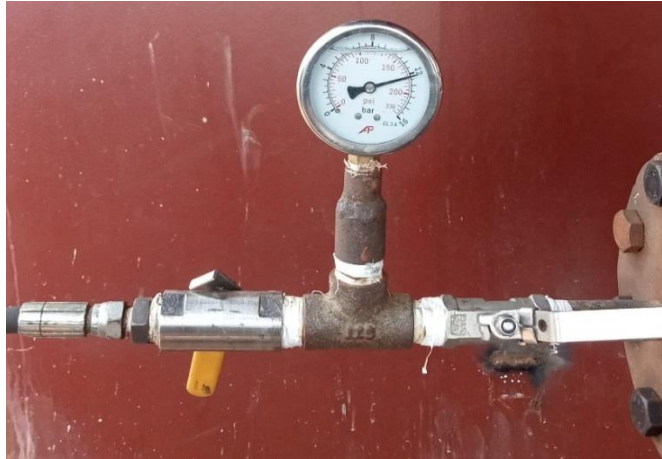
Gambar 2.117 Hydrotest pipe fire
