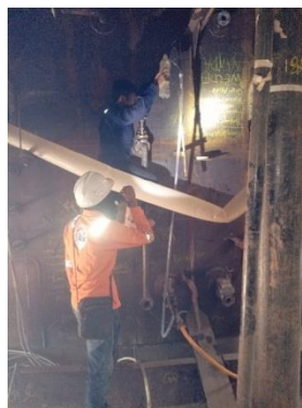
Gambar 2. 33 Pressure airtest tangki Fresh Water
