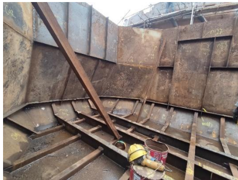
Gambar 2. 89 Visual inspection weal house
