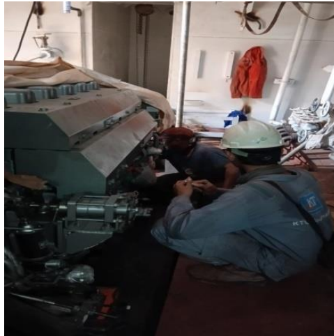
Gambar 2. 56 pengecekan engine room
