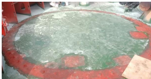
Gambar 2.8 progress fiber manehole area penutup z-peller
