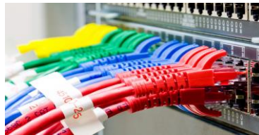
Gambar 3.11 Kabel Wiring Sumber: ( https://i.ytimg.com/ )
