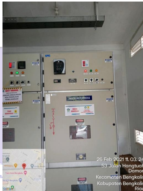
Gambar 2. 7 eviden feeder incoming express (Sumber : Dokumentasi.2021)
