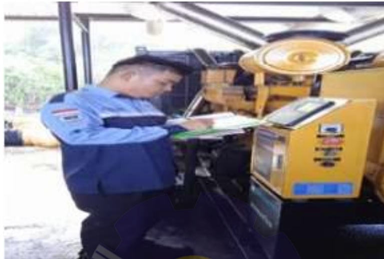
Gambar 2.19 Monitoring Kwh ( Sumber :PT.MEGAPOWER MAKMUR Tbk.2021)
