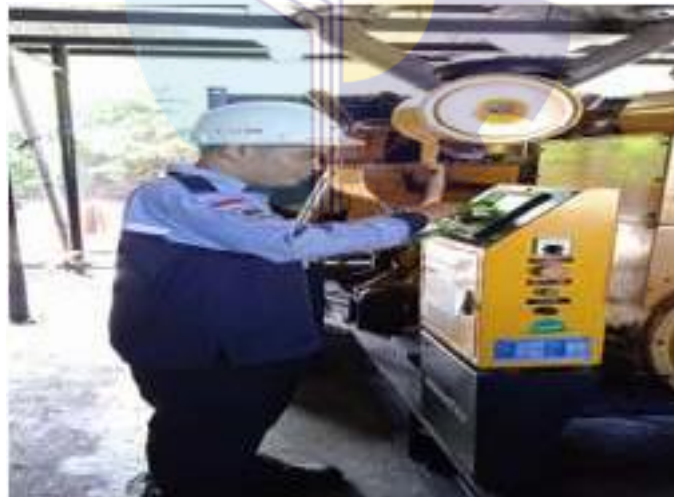
Gambar 2.10 Mnitoring Kwh ( Sumber : PT.MEGAPOWER MAKMUR Tbk.2021)
