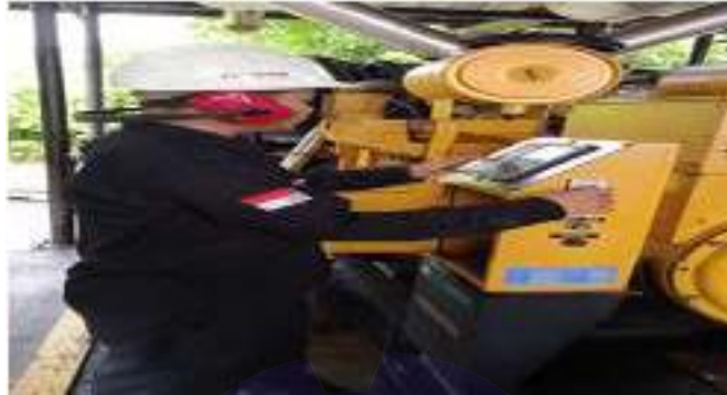
Gambar 2.1 monitoring kwh ( Sumber : PT.MEGAPOWER MAKMUR Tbk.2021)
