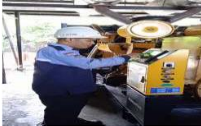
Gambar 2.5 monitoring kwh ( Sumber : PT.MEGAPOWER MAKMUR Tbk.2021)
