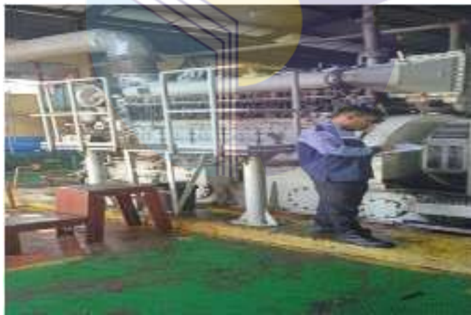
Gambar 2.4 Monitoring kwh ( Sumber : PT.MEGAPOWER MAKMUR Tbk
