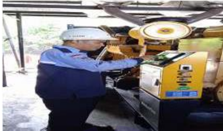
Gambar 2.11 Monitoring Kwh ( Sumber : PT.MEGAPOWER MAKMUR Tbk.2021)
