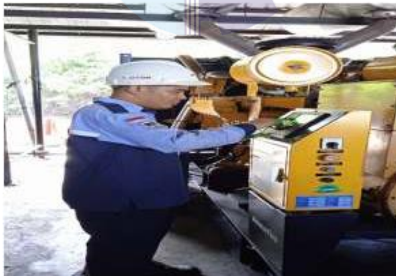
Gambar 2.18 monitoring kwh ( Sumber :PT.MEGAPOWER MAKMUR Tbk.2021)
