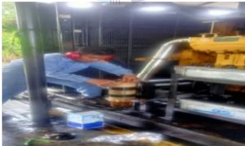
Gambar 2.22 penggantian filter bahan bakar ( Sumber :PT.MEGAPOWER MAKMUR Tbk.2021)
