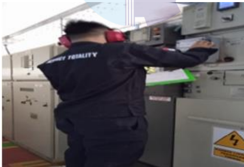
Gambar 2.20 Monitoring kwh ( Sumber :PT.MEGAPOWER MAKMUR Tbk.2021)
