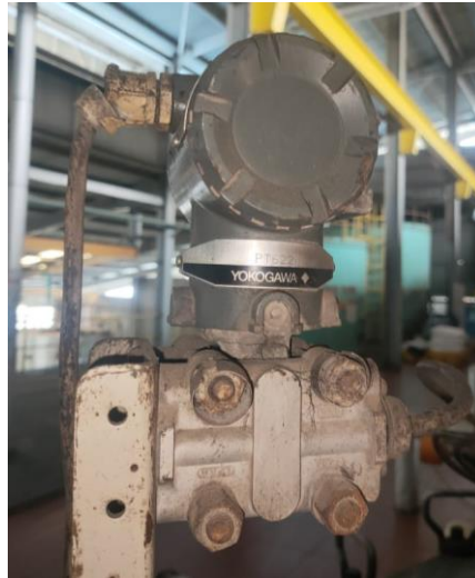
Gambar 3.10 Differential Pressure Transmitter di Wilmar
