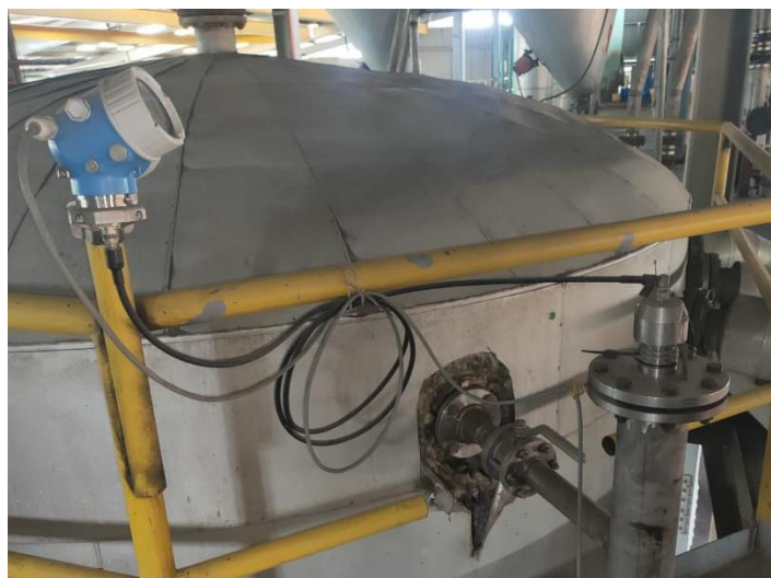
Gambar 3.3. Level transmitter di tangki Crystallizer
