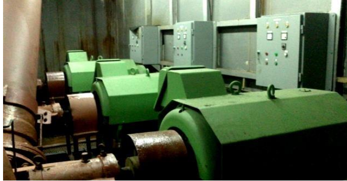
Gambar 1.9 Motor Pompa Graving Dock
