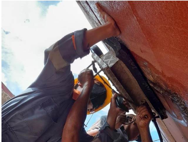
Gambar 2.9 Proses Vacum Test Area Replating Lajur Bilga Bagian Portside Frame No. 60-65 Kapal Trifosa
