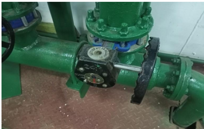
Gambar 2. 52 Valve suction after ballast portside (open)
