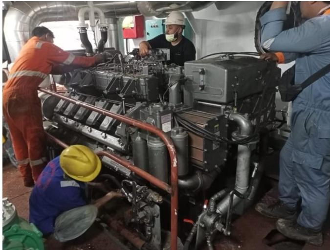
Gambar 2. 54 Commissioning main engine.
