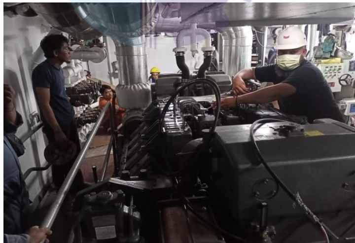
Gambar 2. 55 Sta- up main engine
