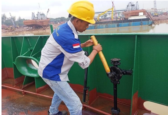
Gambar 2. 48 Commissioning terhadap manual pump chain loker
