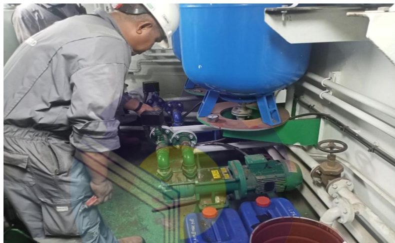
Gambar 2. 63 Commissioning terhadap SW dan FW pressure pump
