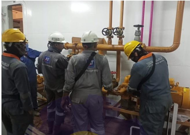
Gambar 2. 18 Pengecekan fuel oil pump
