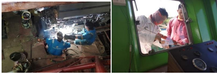
Gambar 2.30 Ruang mesin tugboat repair jendela navigasi tugboat Nelly 19
