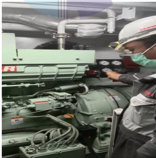
Gambar 2. 37 Commisioning safety device
