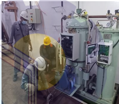
Gambar 3. 1 System oil water separator (OWS)
