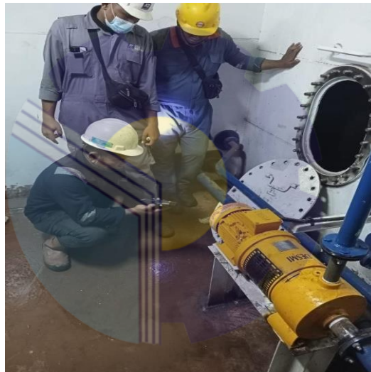
Gambar 2. 17 Commisioning pompa fresh water
