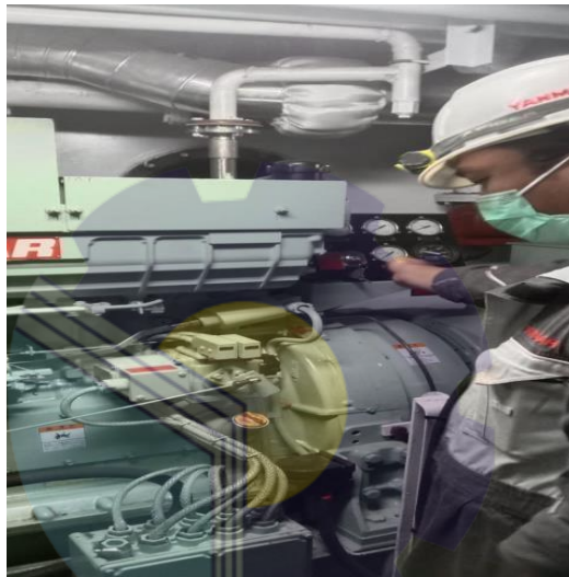
Gambar 2. 37 Commisioning safety device
