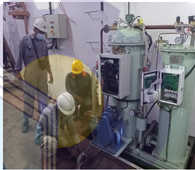
Gambar 3. 1 System oil water separator (OWS)
