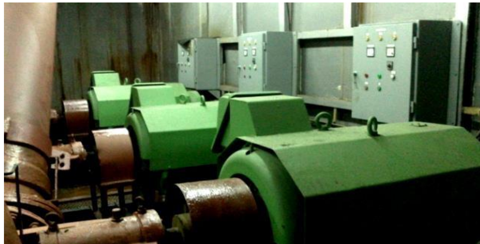
Gambar 1.10 Motor Pompa Graving Dock
