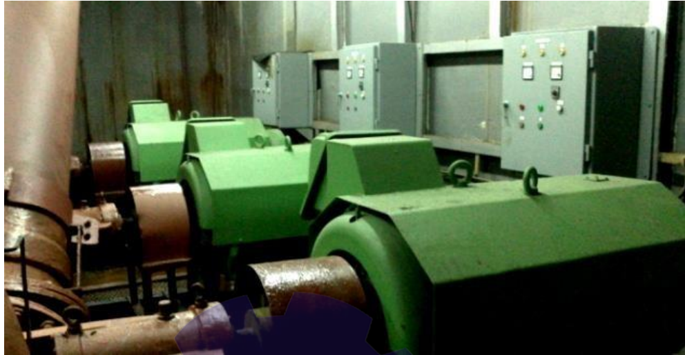
Gambar 1.10 Motor Pompa Graving Dock
