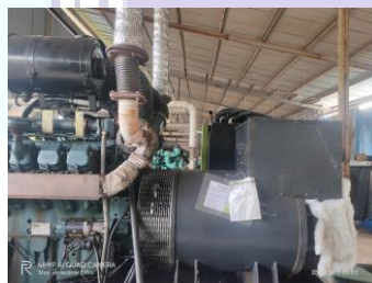
Gambar 3.20 Generator Type Stamford 375 KVA
