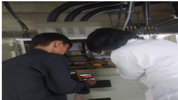
Gambar 2. 59 Maintenance Panel 11 KV switchgear (Sumber: Unit Layanan PLTA Koto Panjang. 2022)
