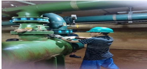
Gambar 2. 12 Maintenance HE (heat exchanger) (Sumber: Unit Layanan PLTA Koto Panjang. 2022)
