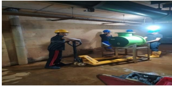
Gambar 2. 22 Maintenance HE (Heat exchanger) (Sumber: Unit Layanan PLTA Koto Panjang. 2022)
