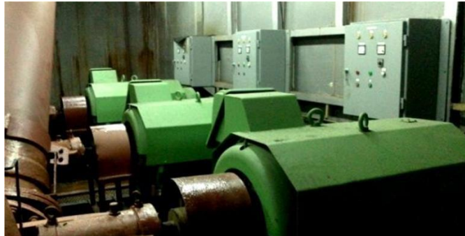
Gambar 1.8 Mesin Pompa Graving Dock
