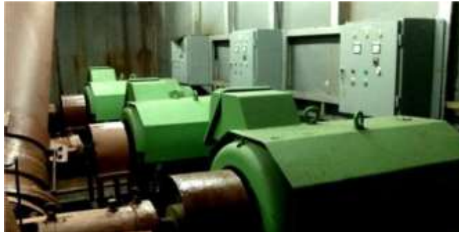
Gambar 1.8 Mesin Pompa Graving Dock
