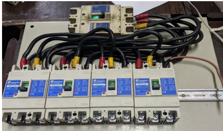
Gambar 3.2 MCCB ( Mold Case Circuit Breaker ) (Sumber: Dokumentasi di PT. Indah Kiat Pulp & Paper)
