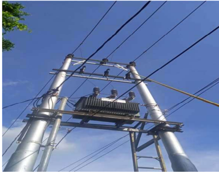
Gambar 2.1 Trafo Distribusi Portal
