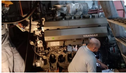
Gambar 2.35 Crank Shaft Deflection after Chockfast (Yanmar)
