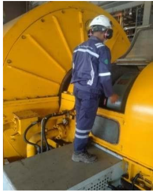
Gambar 2.36. PM Diarea Generator
