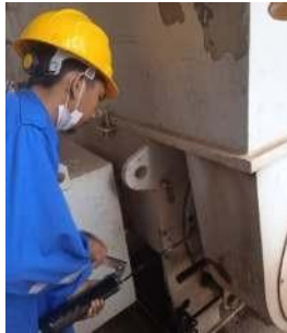
Gambar 2.33. PM Diarea Boiler
