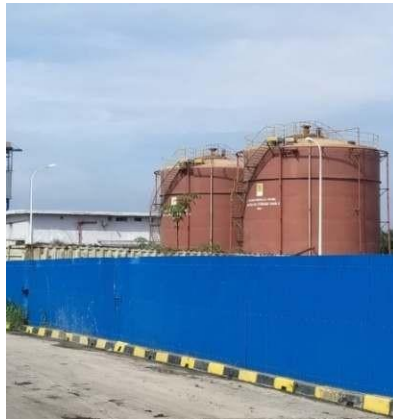
Gambar 1.29. Fuel Oil Tank PLTU Tenayan
