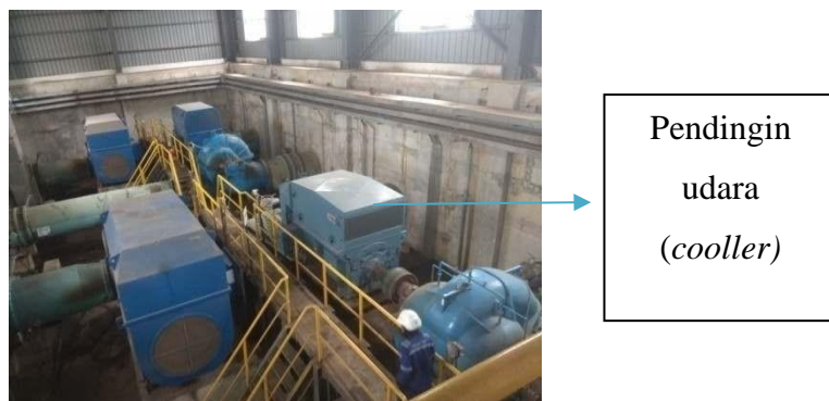
Gambar 3.1 CWP ( Circulating Water Pump ) (Sumber: Dokumentasi di PLTU Tenayan)
