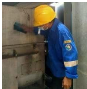
Gambar 2.35. PM Diarea Boiler Motor HPFF 6 kv
