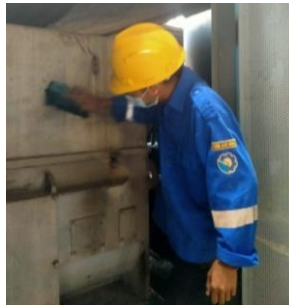
Gambar 2.35. PM Diarea Boiler Motor HPFF 6 kv
