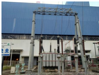
Gambar 2.10. Service Station Transformator
