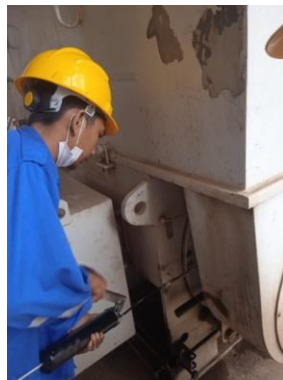
Gambar 2.33. PM Diarea Boiler
