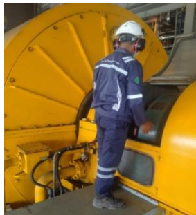
Gambar 2.36. PM Diarea Generator
