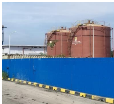
Gambar 1.29. Fuel Oil Tank PLTU Tenayan (Sumber: Dokumentasi di PT PJB UBJOM PLTU Tenayan)
