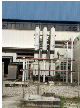
Gambar 2.9. Unit Auxillary Transformator
