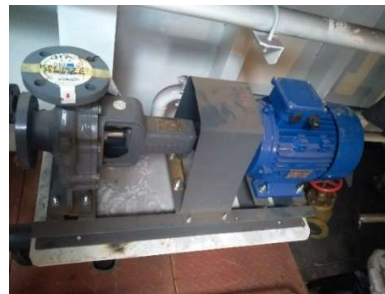
Gambar 3.5 Pompa General Service
