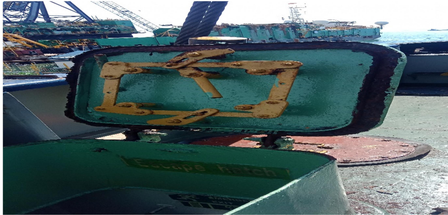
Gambar 2.12 : emergency exit sebelum di reparasi
