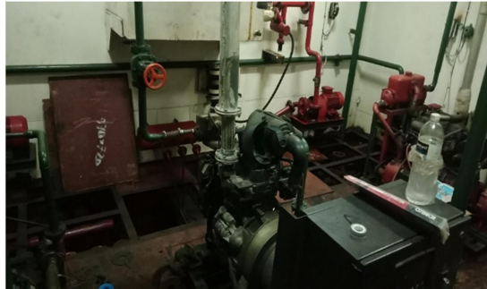
Gambar 2.31 : ruangan engine pompa/diesel pump
