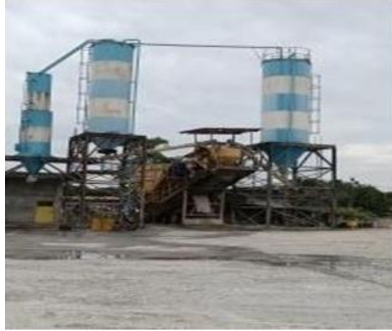
Gambar 1.3. Mesin Batching Plant
