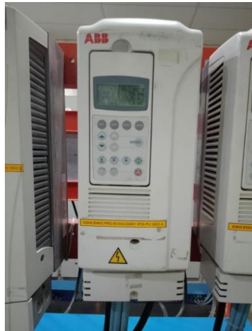
Gambar 2.25 Variable Frequency Drive Sumber : PT. Wilmar Bioenergi Indonesia, (2022)
