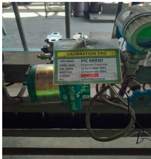
Gambar 2.34 Pressure Transmitter PIC 6893 D Sumber: PT. Wilmar Bioenergi Indonesia, (2022)
