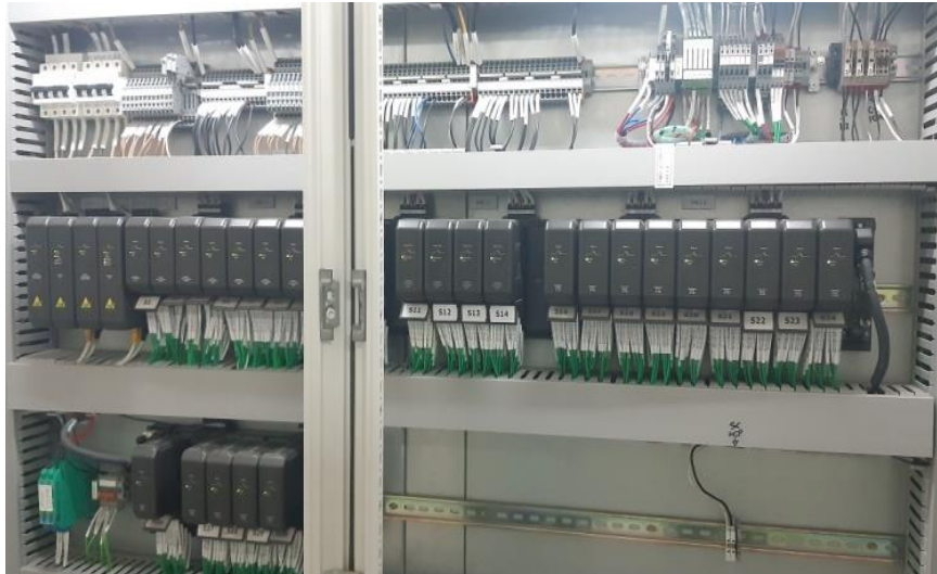
Gambar 3.11 Panel DCS PT. Wilmar Nabati Indonesia Sumber : PT. Wilmar Bioenergi Indonesia, (2022)
