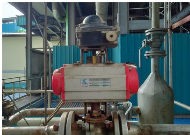
Gambar 2.8 Control Valve Sumber : PT. Wilmar Bioenergi Indonesia, (2022)
