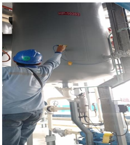
Gambar 2.32 Level Switch LS 10202 Sumber : PT. Wilmar Bioenergi Indonesia, (2022)
