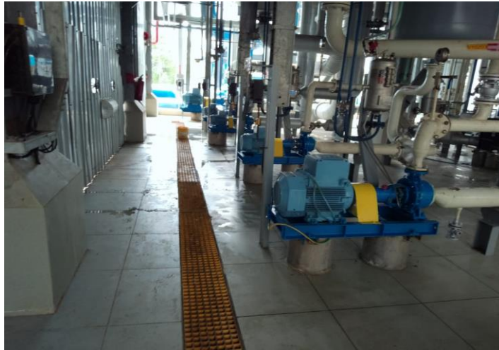
Gambar 2.15 Elektro Motor Plant Enzymatic Sumber : PT. Wilmar Bioenergi Indonesia, (2022)
