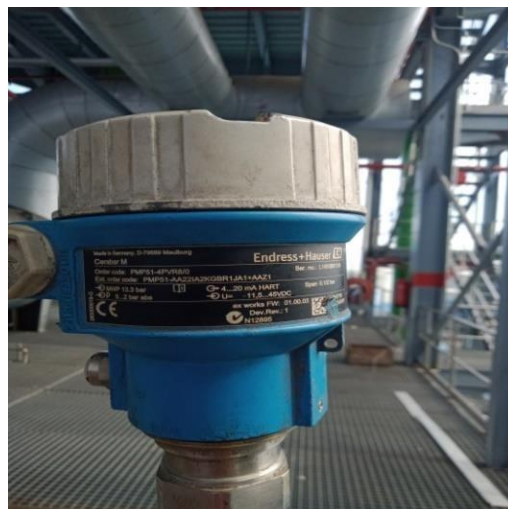
Gambar 2.28 Pressure Transmitter PT 91418 RG 300
