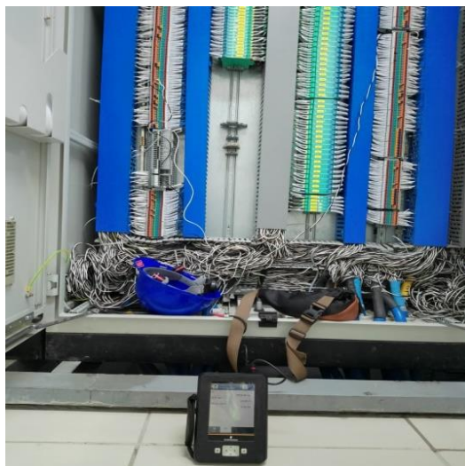
Gambar 2.18 Terminal TB Panel MCC Sumber : PT. Wilmar Bioenergi Indonesia, (2022)
