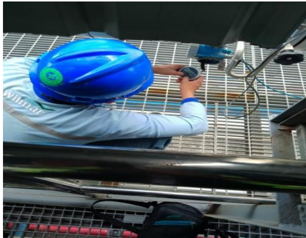
Gambar 2.31 Flowmeter FT 11401 Sumber : PT. Wilmar Bioenergi Indonesia, (2022)
