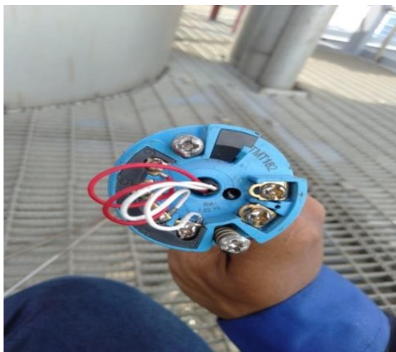
Gambar 2.14 Temperature Transmitter Sumber : PT. Wilmar Bioenergi Indonesia, (2022)
