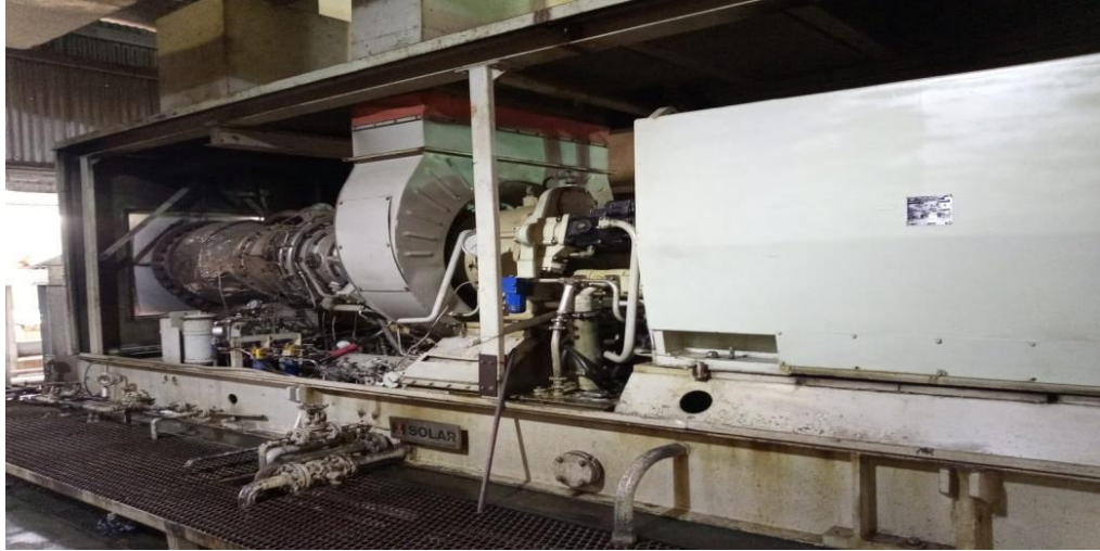
Gambar 3.2 turbin gas generator
