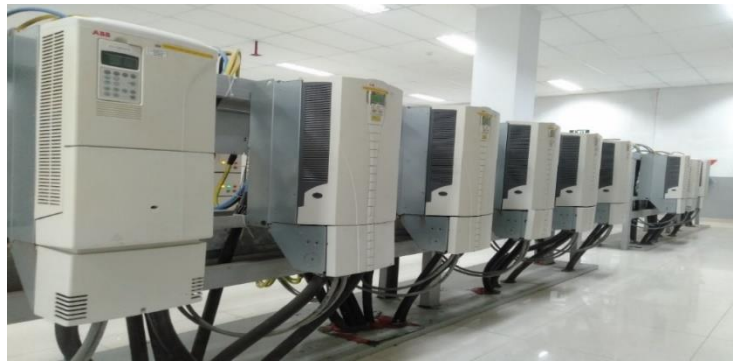
Gambar 3. 4 Panel Inverter (Sumber: PT. WINA OLEO CHEMICAL, 2022)
