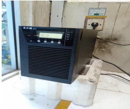
Gambar 2. 24 Ups (Uninterrubtible Power Supply) (Sumber: PT. WINA OLEO CHEMICAL, 2022)
