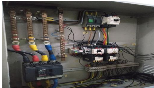
Gambar 2. 34 Instalasi Rangkain Star Delta (Sumber: PT. WINA OLEO CHEMICAL, 2022)
