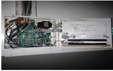
Gambar 2. 1 Instalasi Kontrol Fire Alarm (Sumber: PT. WINA OLEO CHEMICAL, 2022)
