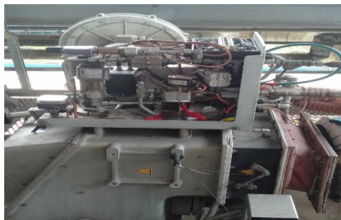
Gambar 2. 30 Burner (Sumber: PT. WINA OLEO CHEMICAL, 2022)
