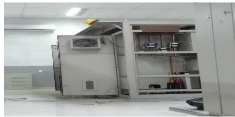
Gambar 2. 6 Servis Panel Mcc (Sumber: PT. WINA OLEO CHEMICAL, 2022)
