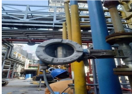
Gambar 2. 27 Pengecekan Flow Meter (Sumber: PT. WINA OLEO CHEMICAL, 2022)
