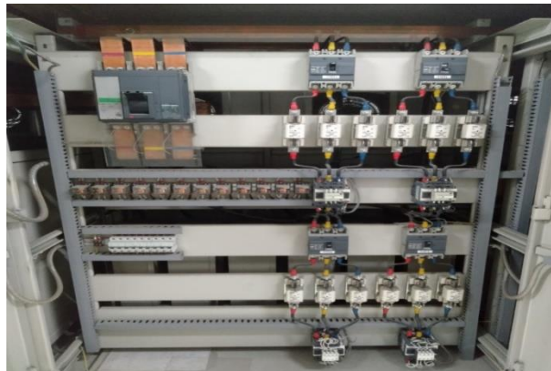
Gambar 3. 6 Panel Kapasitor Bank (Sumber: PT. WINA OLEO CHEMICAL, 2022)
