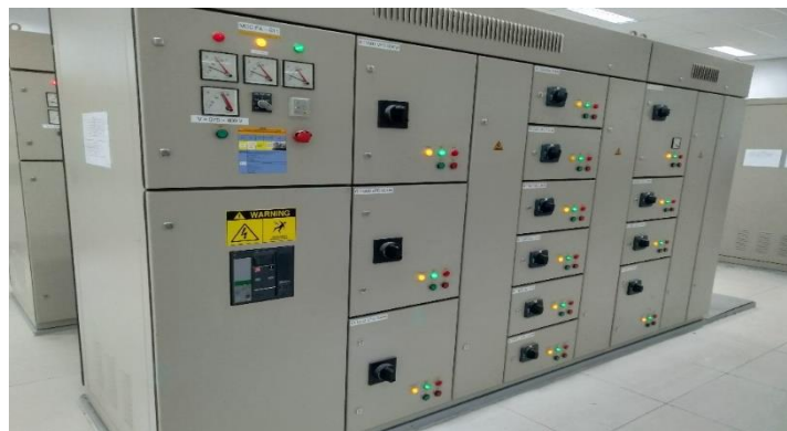
Gambar 3. 3 Panel MCCP (Sumber: PT. WINA OLEO CHEMICAL, 2022)
