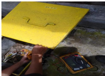
Gambar 2. 42 Pengecekan Kabel Grounding (Sumber: PT. WINA OLEO CHEMICAL, 2022)
