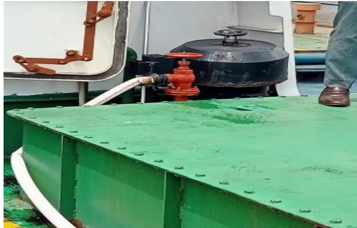
Gambar 2.7 Pengecekan Hydrant Kapal
