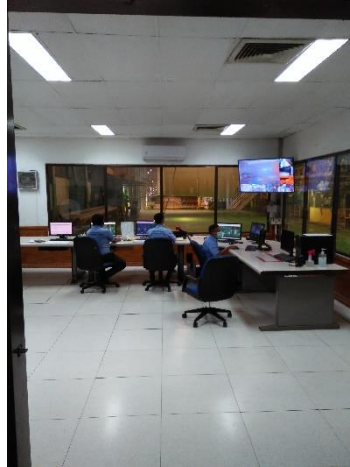
Gambar 3.23 Operator Station (Sumber : Dokumentasi PT. Indah Kiat pulp & paper Tbk Perawang, 2022)
