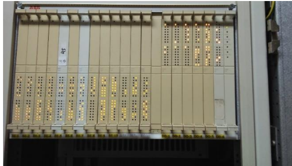
Gambar 3.8 System I/O S100
