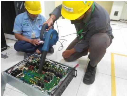
Gambar 2.7 maintenance cleaning UPS (Sumber : Dokumentasi PT. Indah Kiat pulp & paper Tbk Perawang, 2022)
