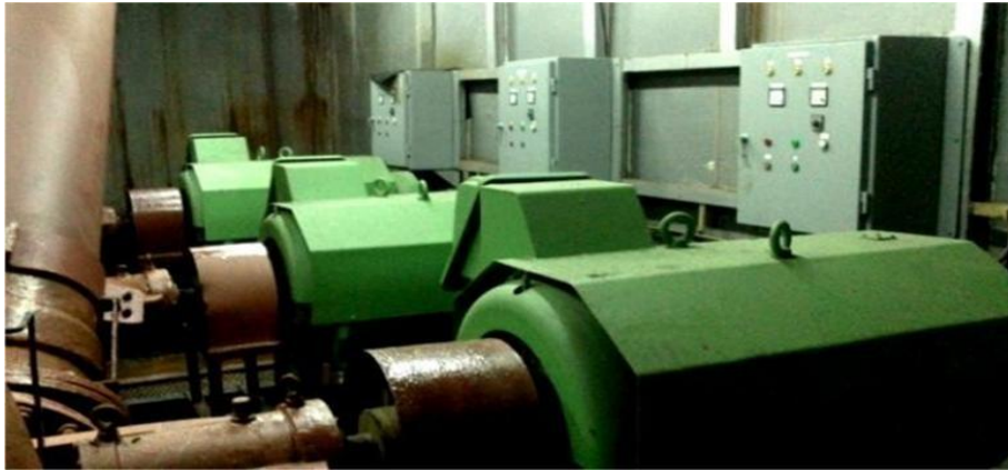
Gambar 1.10 motor pompa Graving dock
