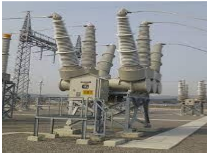
Gambar 3.2 SF6 CB ( Sulfur Hexafluoride Circuit Breaker ) Sumber : Google
