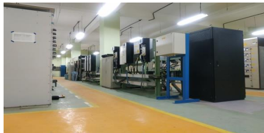
Gambar 2.3 Motor Control Center
