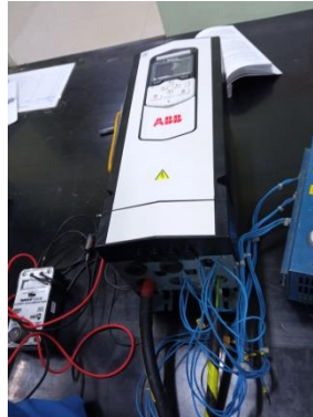
Gambar 2. 8 pengoperasian Variable Speed Drive ACS-880
