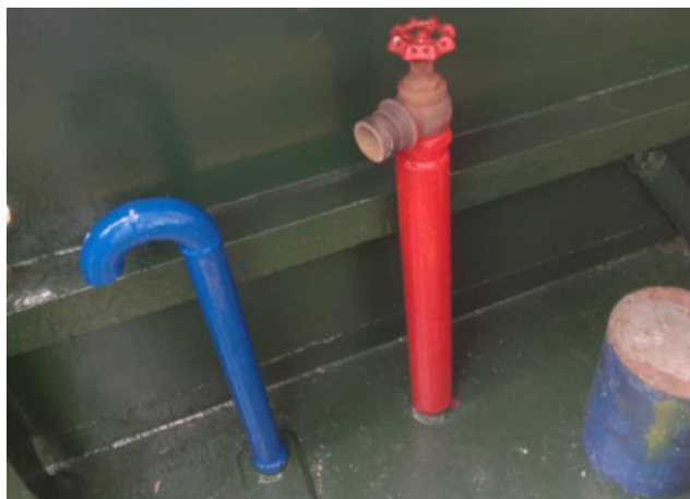
Gambar 3.10 Fire hydrant Kapal Tunda Tinju
