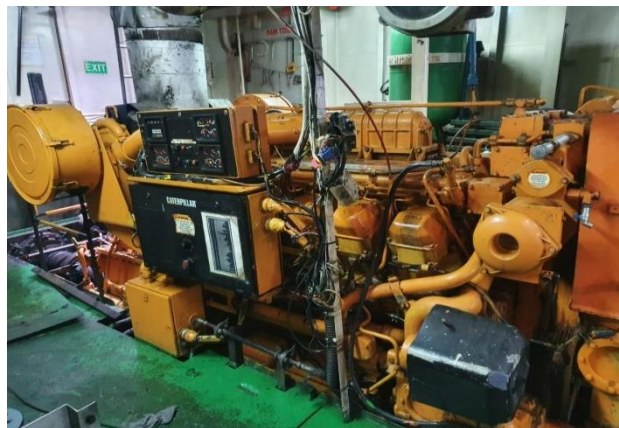
Gambar 3.12 Generator Set Kapal Tunda Tinju
