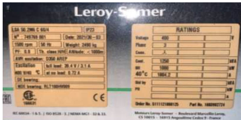
Gambar 3.4 Name Plate Generator 4
