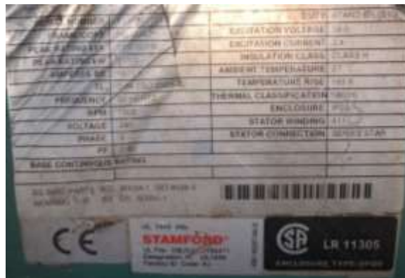
Gambar 3.3 Name Plate Generator 3
