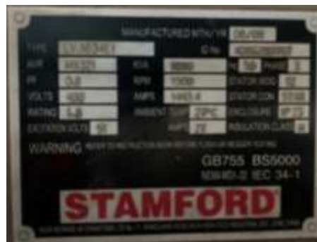
Gambar 3.2 Name Plate Generator 2
