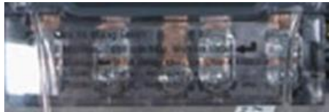
Gambar 3.6. Terminal Block (Sumber: PT. Haleyora Power, 2022)
