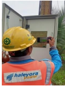
Gambar 2.29. Recloser(Rc) Trip (Sumber: PT. Haleyora Power, 2022)
