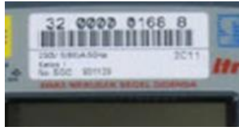
Gambar 3.1. Name Plate (Sumber: PT. Haleyora Power, 2022)
