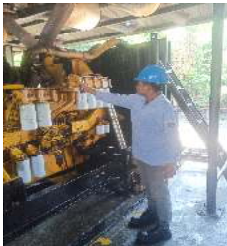
Gambar 2.39 Monitoring KWH (Sumber: PT. Megapower Makmur Tbk. 2022)
