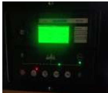
Gambar 2.5 Monitoring KWH (Sumber: PT. Megapower Makmur Tbk. 2022)
