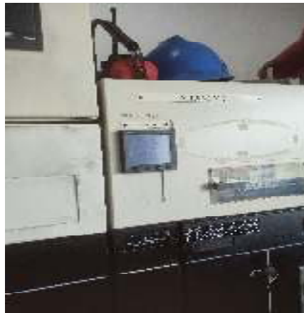
Gambar 2.35 Monitoring KWH (Sumber: PT. Megapower Makmur Tbk. 2022)
