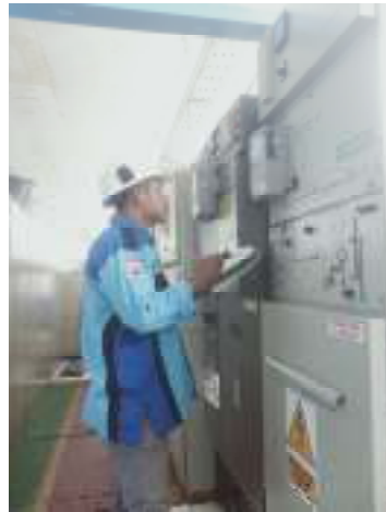
Gambar 2.33 Monitoring KWH (Sumber: PT. Megapower Makmur Tbk. 2022)
