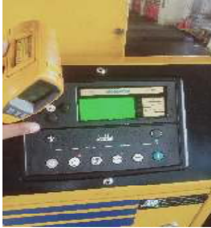
Gambar 2.36 Monitoring KWH (Sumber: PT. Megapower Makmur Tbk. 2022)
