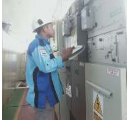
Gambar 2.16 Monitoring KWH (Sumber: PT. Megapower Makmur Tbk. 2022)
