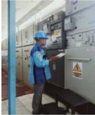
Gambar 2.24 Monitoring KWH (Sumber: PT. Megapower Makmur Tbk. 2022)
