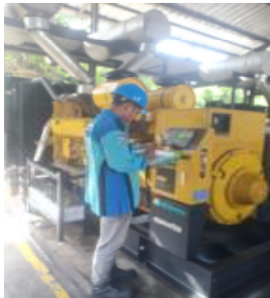
Gambar 2.37 Monitoring KWH (Sumber: PT. Megapower Makmur Tbk. 2022)
