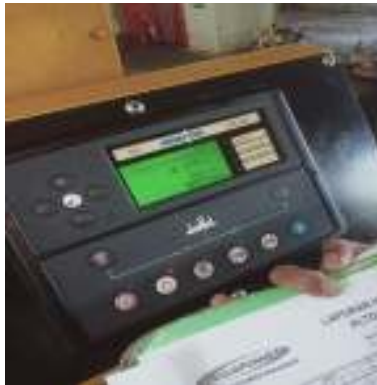
Gambar 2.9 Monitoring KWH (Sumber: PT. Megapower Makmur Tbk. 2022)
