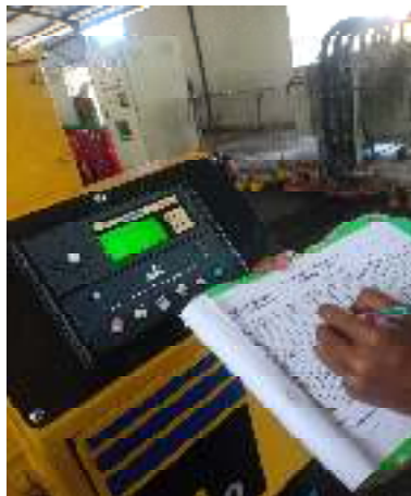
Gambar 2.3 Monitoring KWH (Sumber: PT. Megapower Makmur Tbk. 2022)
