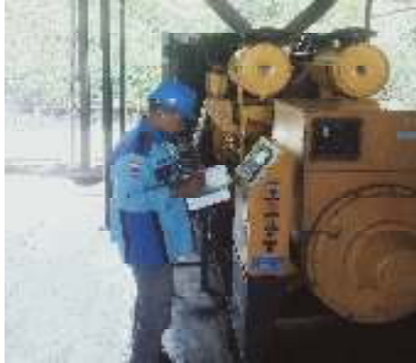
Gambar 2.22 Monitoring KWH (Sumber: PT. Megapower Makmur Tbk. 2022)
