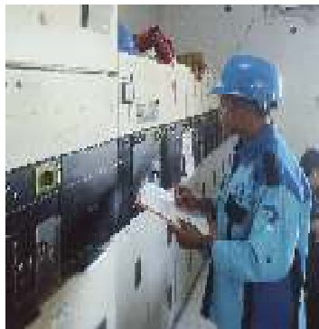
Gambar 2.23 Monitoring KWH (Sumber: PT. Megapower Makmur Tbk. 2022)
