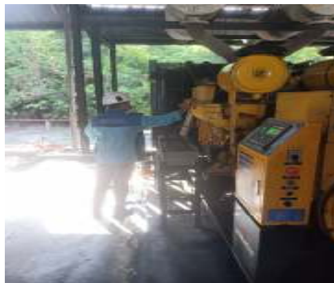
Gambar 2.27 Monitoring KWH (Sumber: PT. Megapower Makmur Tbk. 2022)
