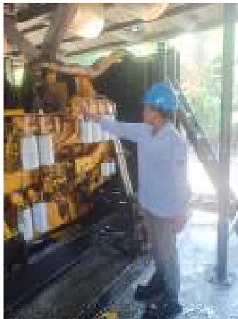
Gambar 2.31 Monitoring KWH (Sumber: PT. Megapower Makmur Tbk. 2022)
