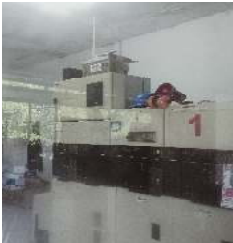
Gambar 2.43 Monitoring KWH (Sumber: PT. Megapower Makmur Tbk. 2022)
