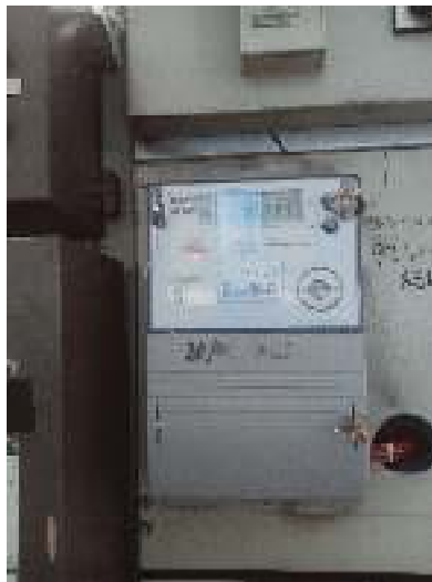
Gambar 2.17 Monitoring KWH (Sumber: PT. Megapower Makmur Tbk. 2022)
