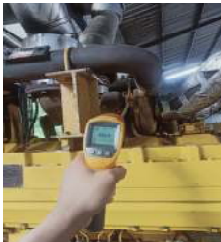
Gambar 2.41 Monitoring KWH (Sumber: PT. Megapower Makmur Tbk. 2022)
