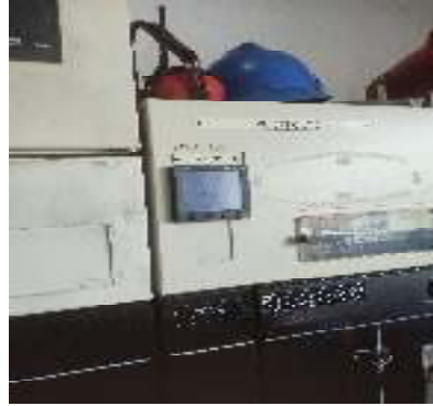
Gambar 2.40 Monitoring KWH (Sumber: PT. Megapower Makmur Tbk. 2022)
