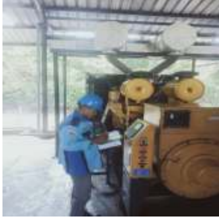
Gambar 2.8 Monitoring KWH (Sumber: PT. Megapower Makmur Tbk. 2022)
