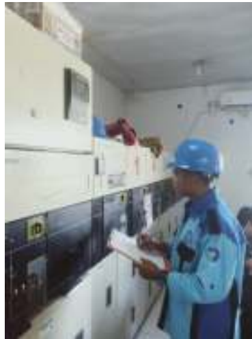
Gambar 2.10 Monitoring KWH (Sumber: PT. Megapower Makmur Tbk. 2022)
