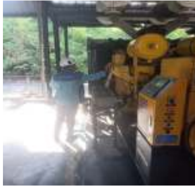
Gambar 2.12 Monitoring KWH (Sumber: PT. Megapower Makmur Tbk. 2022)
