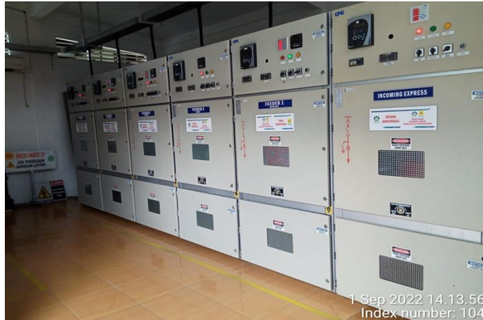
Gambar 2.38 Evident Beban Feeder
