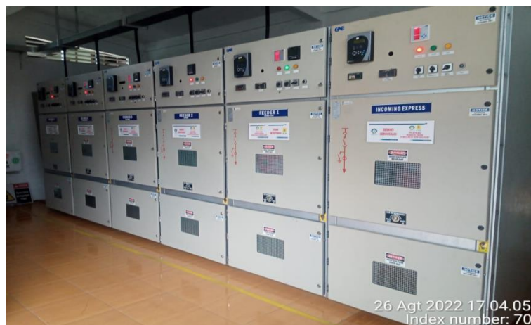
Gambar 2.35 Evident Beban Feeder
