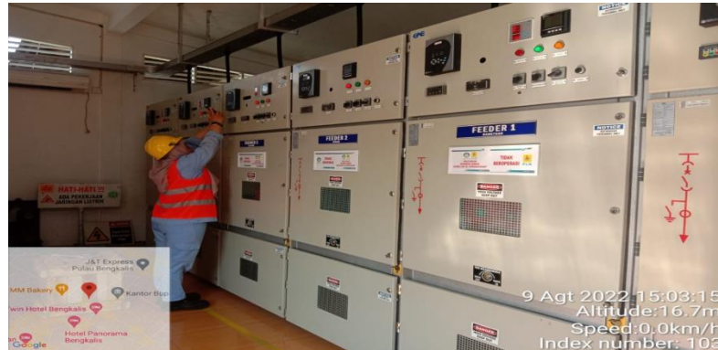
Gambar 2.22 Evident Beban Feeder
