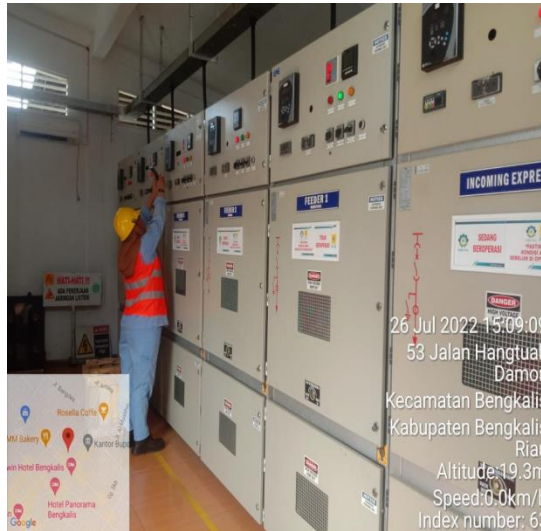
Gambar 2.11 Evident Beban Feeder
