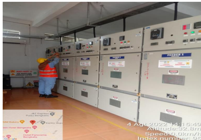
Gambar 2.19 Evident Beban Feeder
