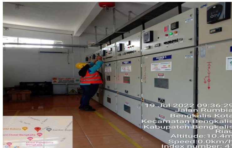
Gambar 2.7 Evident Beban Feeder
