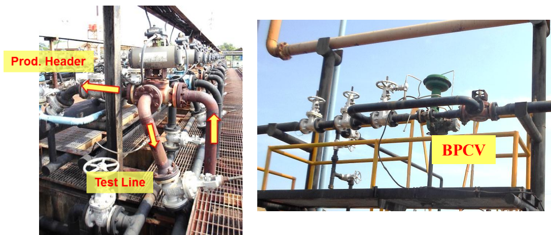
Gambar 3. 3 (a) Prod. Header (b) Test Line (c) BPCV (Sumber: Power Point, 2022)
