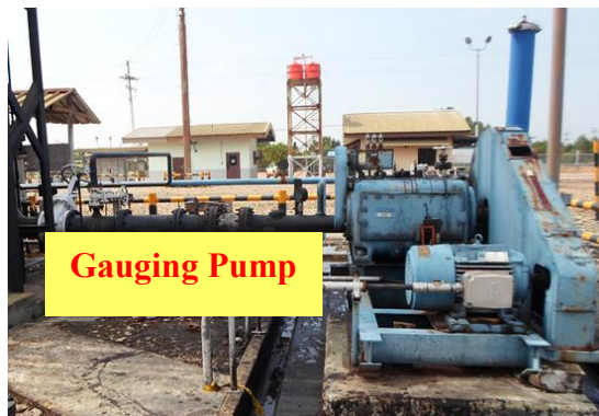
Gambar 3. 4 Gauging Pump (Sumber: Power Point, 2022)
