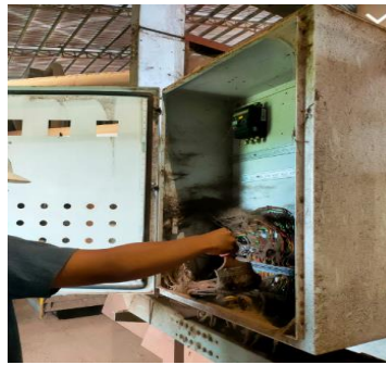
Gambar 2. 2 Maintenance Panel (Sumber: Dokumentasi, 2022)
