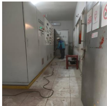
Gambar 2. 16 Maintenance Panel Control (Sumber: Dokumentasi, 2022)
