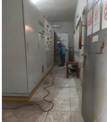
Gambar 2.15 Maintenance panel control (Sumber: dokumentasi, 2022)
