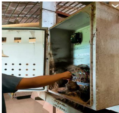
Gambar 2. 2 Maintenance panel (Sumber: dokumentasi, 2022)
