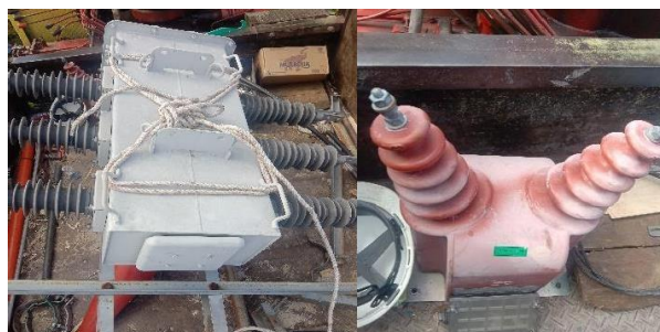
Gambar 2. 1 load break switch (LBS) (sumber: dokumentasi, 2022)
