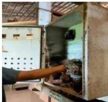
Gambar 2.2 Photo maintenance panel (Sumber:dokumentasi, 2022)
