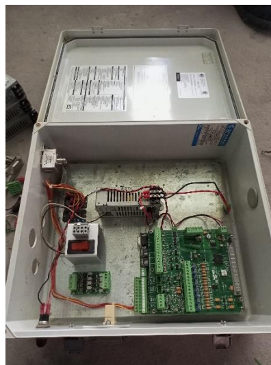
Gambar 3.4 RTU (Remote Terminal Unit) Sumber : PT.Mobilkom Telekomindo
