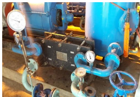
Gambar 4. 3 Heat Exchanger Type Plate and Gasket (Sumber : Dokumentasi Pribadi)
